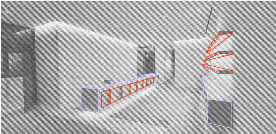
Fig. 18 Detailed and precise pre-planning and prefabrication enable fast and clean work on the construction site.
