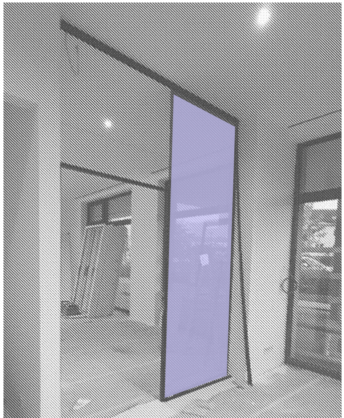
Fig. 21 Installation of glass partitions — precise planning and an exact plan approval process guarantee waste avoidance.
