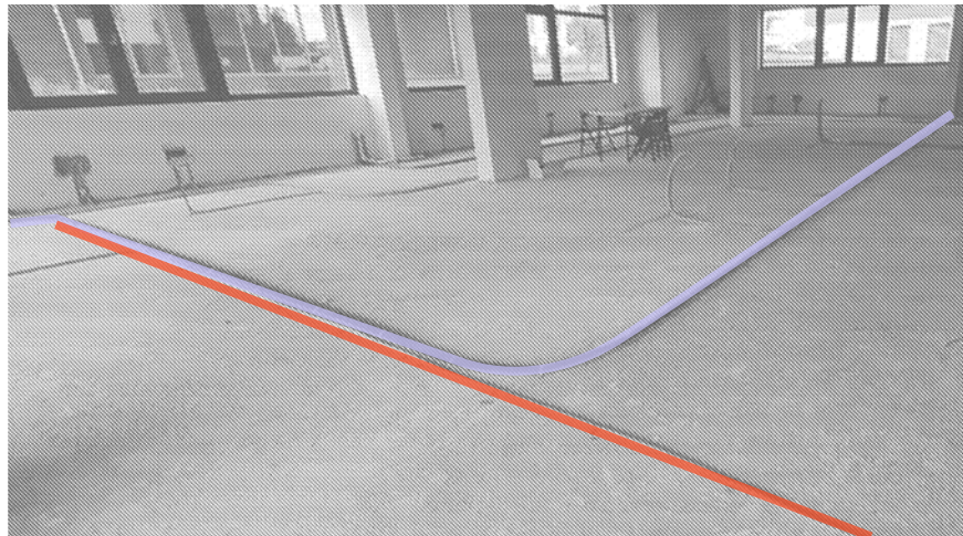
Fig. 03 Electrical installation Pre-assembly of cable lengths enables precise work on the construction site
